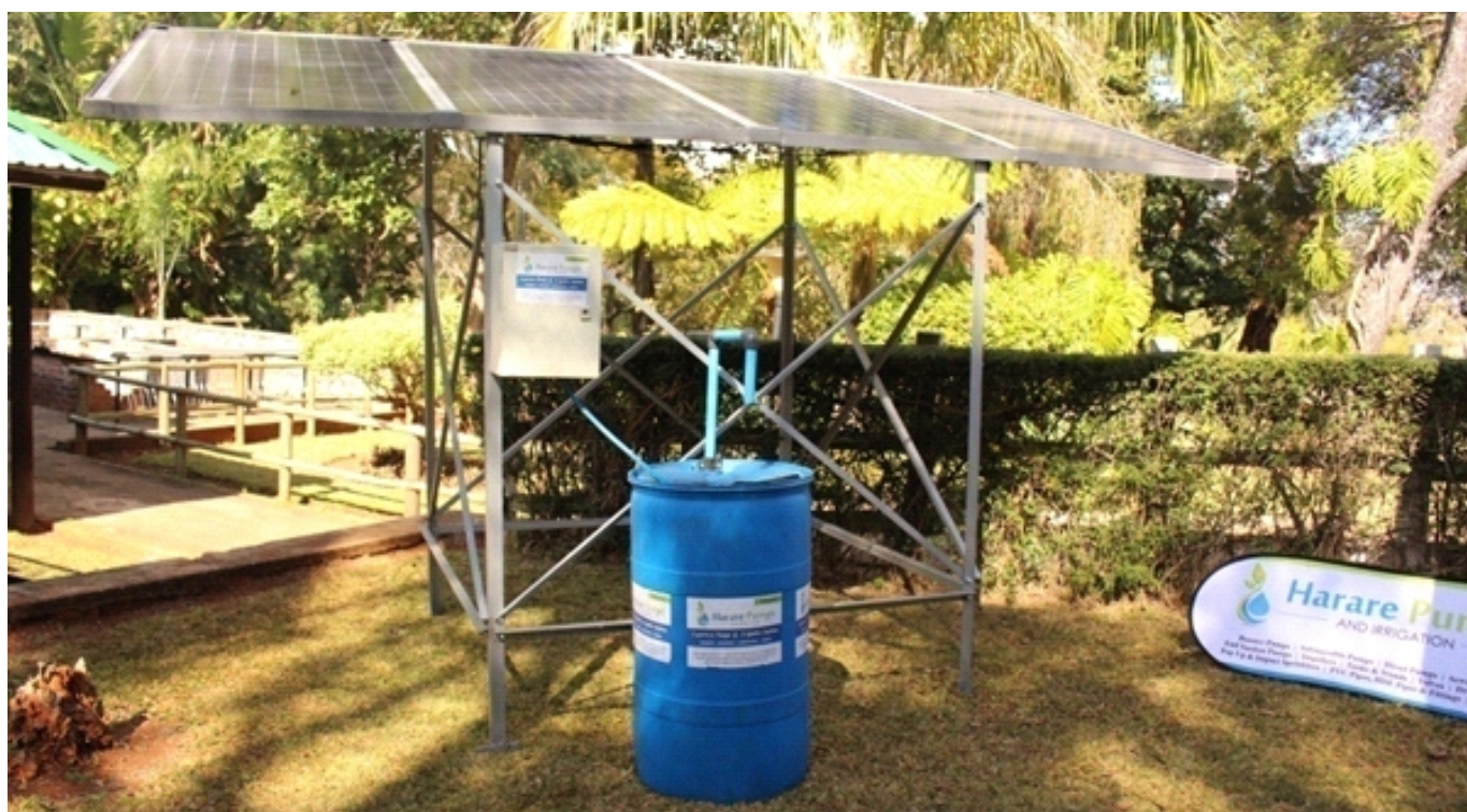
A solar borehole system on exhibition at a reflection workshop, Wise Owl Motel, Mutare
