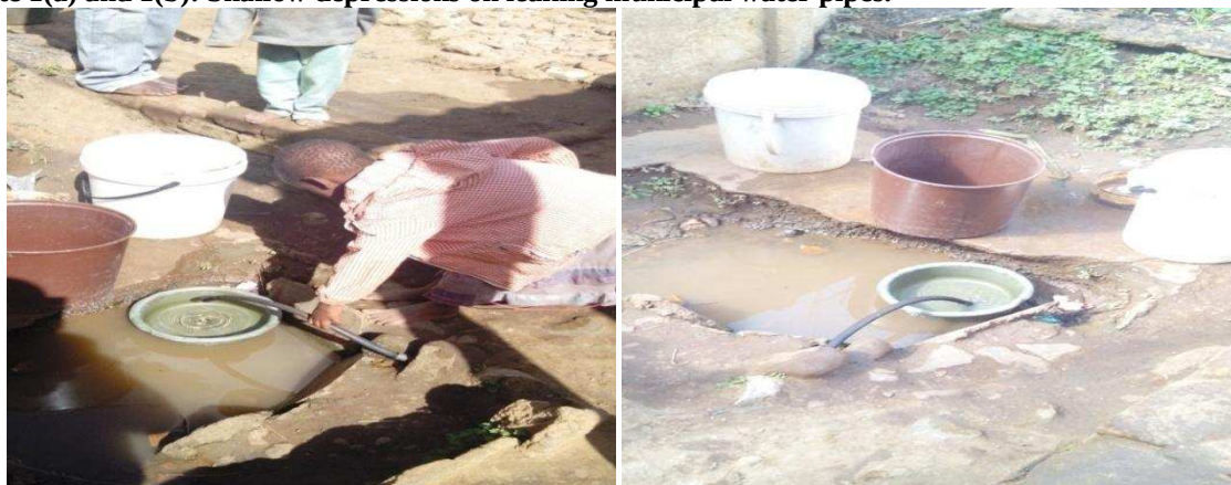
Plate 1(a) and 1(b): Shallow depressions on leaking municipal water pipes.
